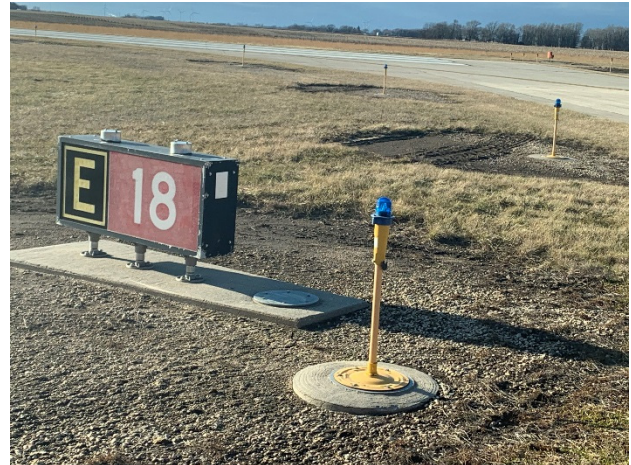
Airfield Signage and Taxiway Lighting
